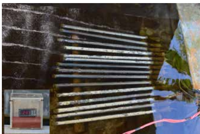
Water heaters installed near the sand filter tank
