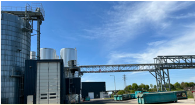
The 300m pipeline that feeds the stillage which is 80% water and bran from Tereos to Innovafeed into storage tanks with mixers operable in real-time to get the right mix of feed substrate.
