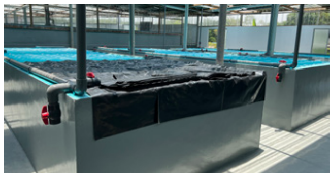
New larval rearing tanks to cater for an expansion in production to 20 million PL10/month by 2024.
