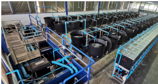
Figure 4. View of RAS and testing facilities at Aqualis APAC
