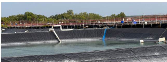
Incoming water slowly moves around baffles, settling organic matter. In the final treatment pond, chlorine gas is added.
