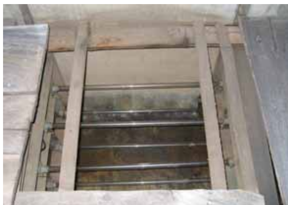
Hendra has installed 210 UV lamps over a 30 metres stretch of cement lined canal to eliminate disease carriers in incoming water.
