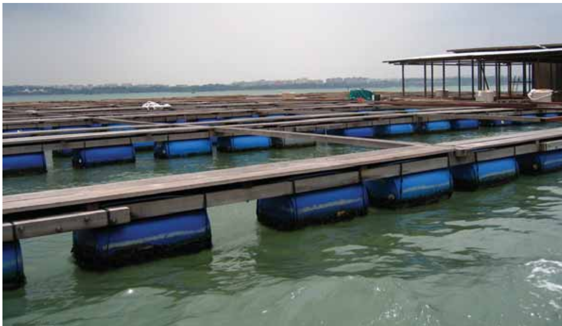
Some 108 units of cages are being installed off Pulau Ubin in Singapore. The expected production will be one tonne per cage. The total production per cycle will be 60 tonnes as 20% of the cages will be used as nursery cages.
