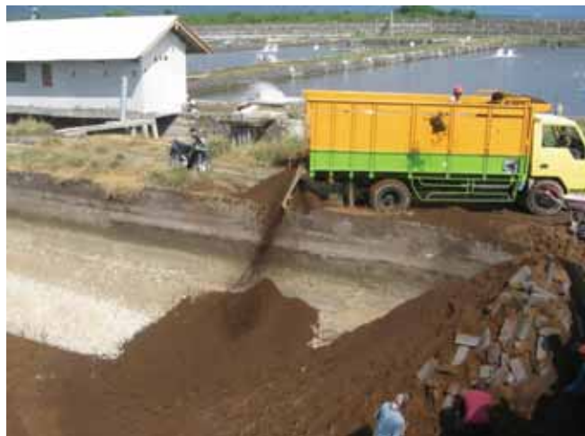
Old pond bottom soil is replaced by new soil before each cycle.
