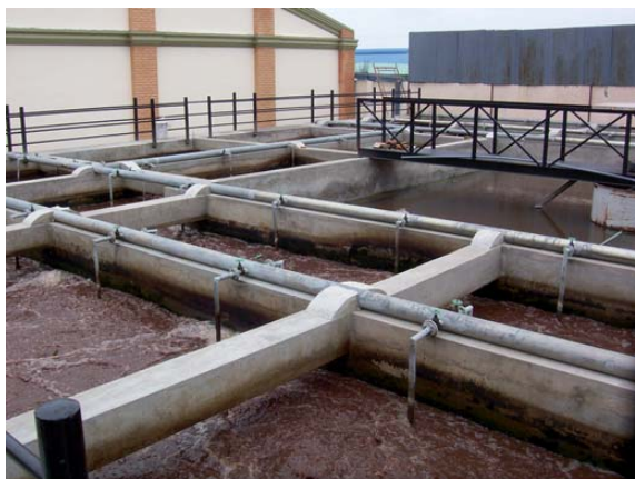
Large processing plants invest in water purification systems such as above.
