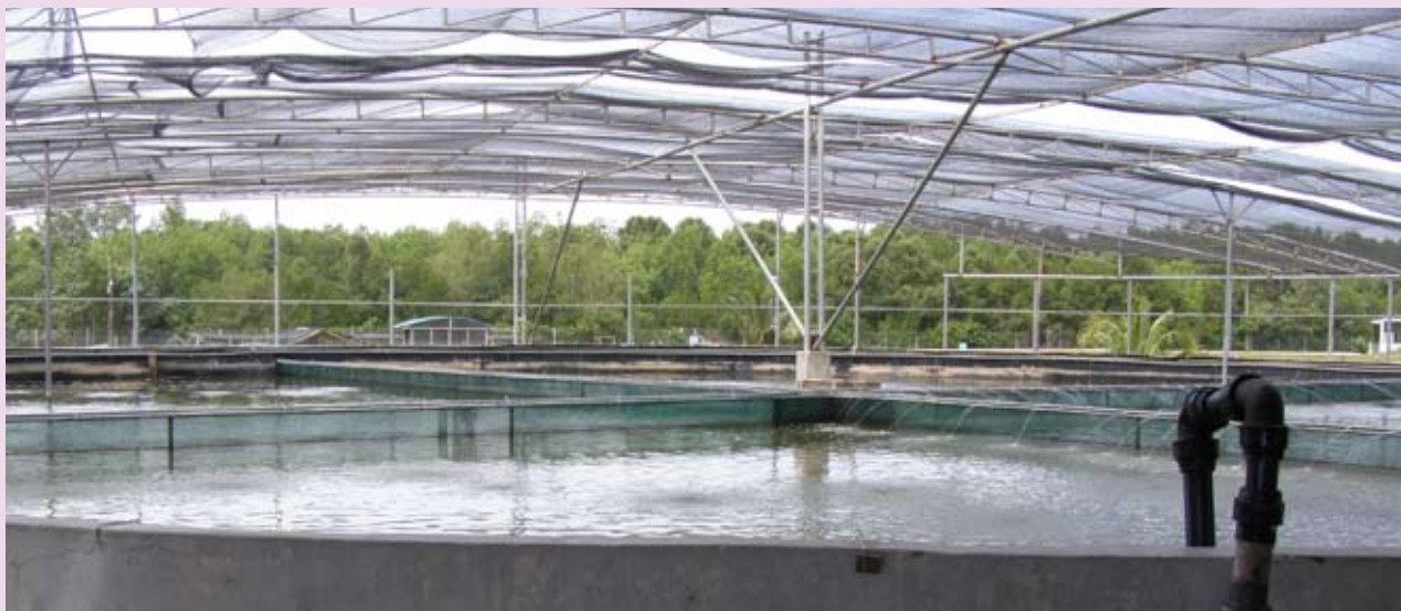
Indoor brood stock tanks. Water from the main reservoir of 4 ha goes to a sedimentation pond and biological filter before being subjected to chlorine treatment, biological and mechanical filtration and finally is UV treated separately at the five modules of the centre.
