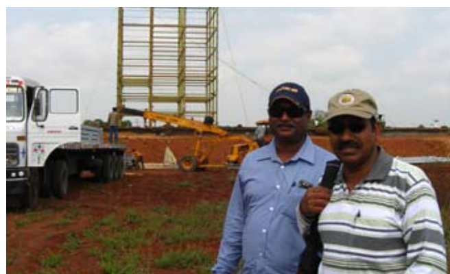
A new plant with a 10 tph Extru-Tech extruder for Rudra Techno Feeds.
