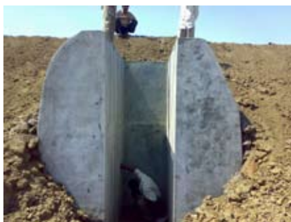
A constructed pond indicating depth at outlet
