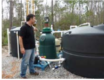
A new facility designed to recover the marine salt from the waste water because they are using expensive artificial salt in all their research facilities.
