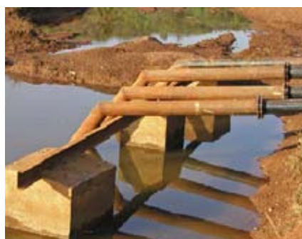
Source of water is the dumping ground of waste discharge
