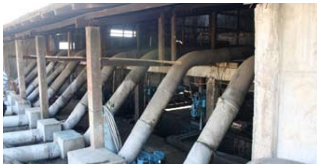
The pump station for intake water
