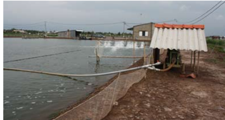
Pumping station for diffused aeration system
