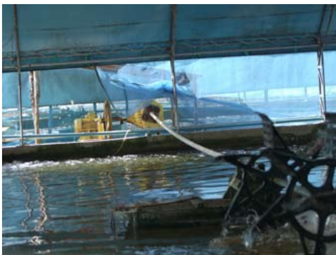
This 5HP source drives paddlewheels in the cement ponds.
