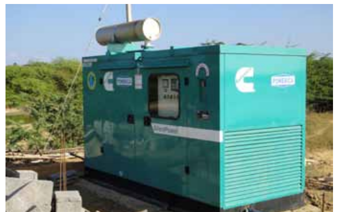
The recently installed generator set
