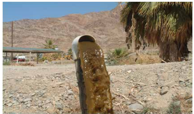
Drain bottom sludge twice daily till you get clear water
