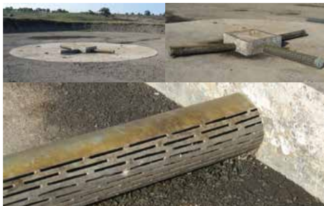
Photos showing central sludge removal system
