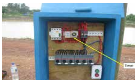
A timer-starter allows phased starting of sets of aerators.
