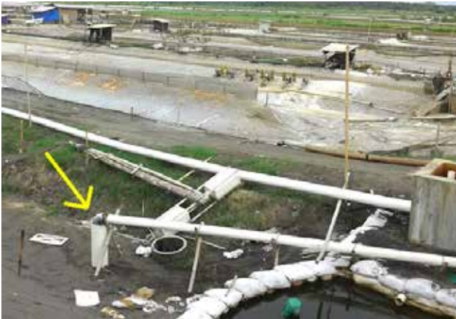
A 6-inch (15.2 cm) pump in an 8-inch (20 cm) casing at about 8 m deep supplying filtered sea water to the ponds
