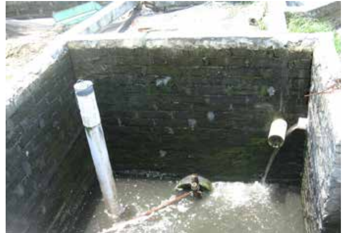
This sump receives outlet water from several ponds, the water then drains away via a 75 cm diameter culvert buried 15 cm below the pond bottom level.
