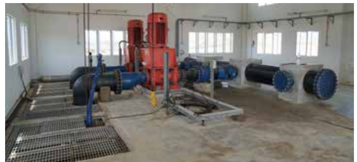
Pumps in the marine outfall station
