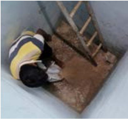
A nursery staff demonstrates how the sludge is removed from the large 150-tonne tank. Sludge removal is carried out every 12 hours
