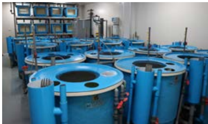
Recirculating rearing system
