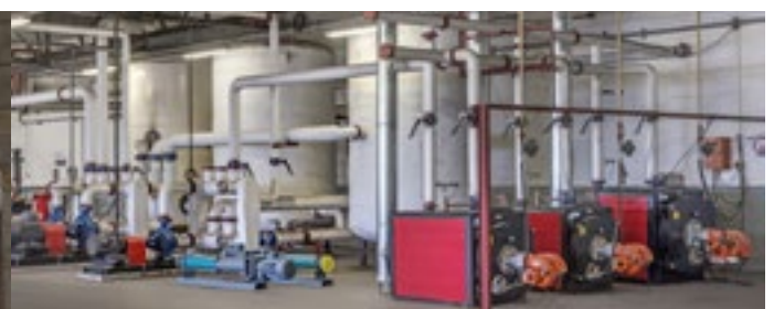
Boilers used to keep factory warm and at the right temperatures for larvae growth. Photo credit: AgriProtein
