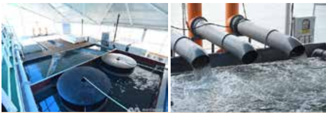
Water treatment systems. Right, three pumps located in the bow section of the hull, designed to have a low pumping height are very cost and energy efficient and on the left, ozone generators.
