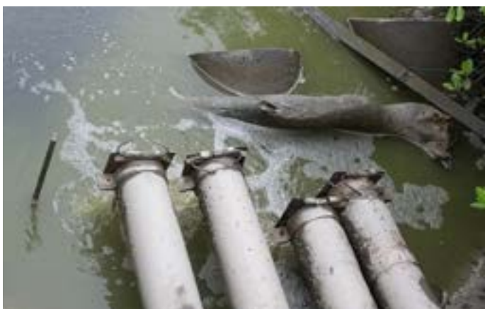
Series of automatic check valve to discharge outlet water during low tide but closes automatically when the tide rises.
