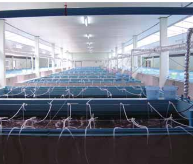
The hatchery at the Sureerath farm with insulated piping
